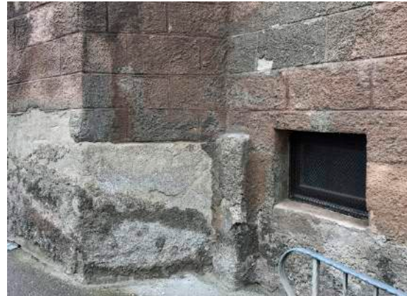
Damage patterns such as salt efflorescences and damp stains
