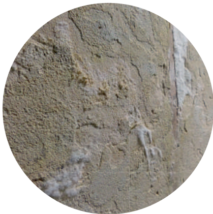
Spalling and salt efflorescences; high salt pressure
